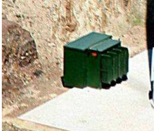
Figure 6. Indicative transformer structure associated with each turbine of the type proposed in the TRHE.
